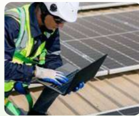
Solar PV Installation for Suppliers
